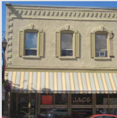
Narrow shutters are not in scale with window width and appear to be inoperable.
