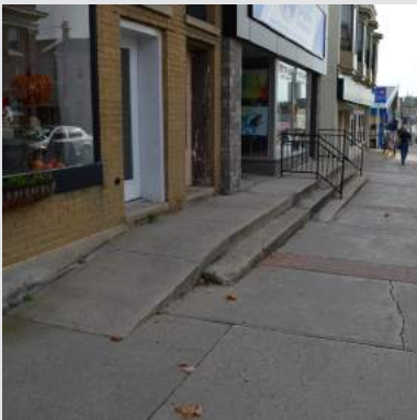
Ramps without handrails provide obvious challenges.
