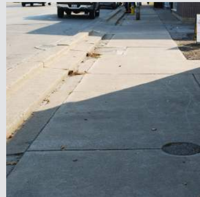
Uneven paving and obstructed sidewalk provide additional obstacles.
